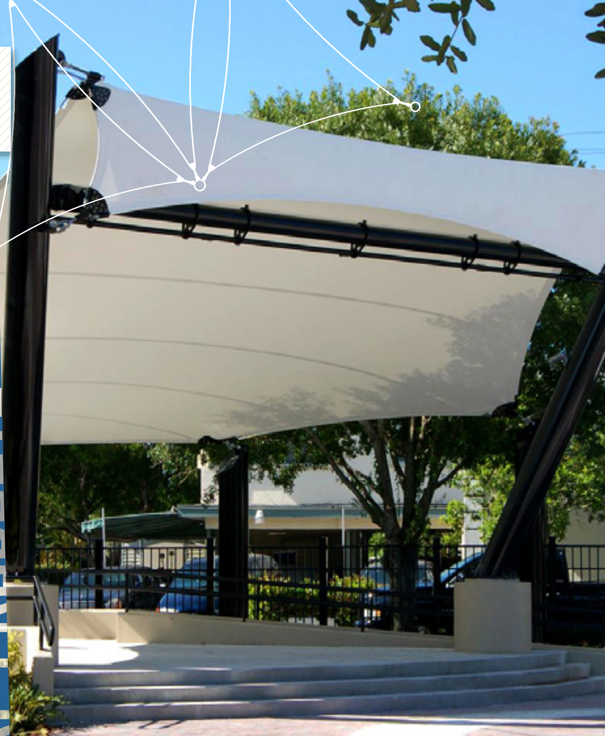
Custom Tension Shade Structure
